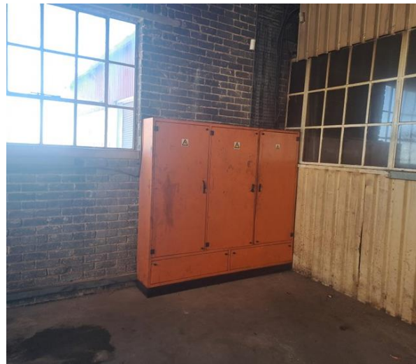
PHOTOGRAPH 3-8: Photograph showing existing electrical distribution box.
