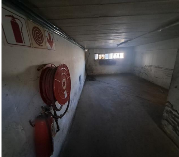
PHOTOGRAPH 3-7: Photograph showing existing firefighting equipment.
